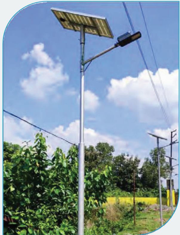
(Solar Street Light)
